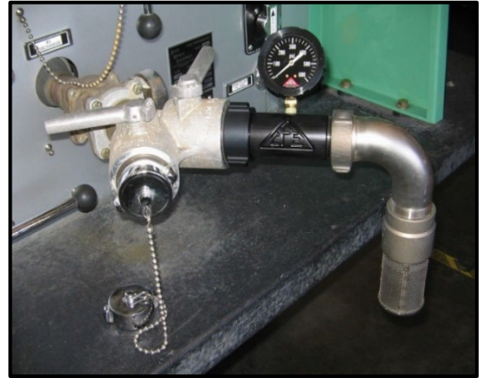
Figure 12: Pressure valve attached to the foot valve
